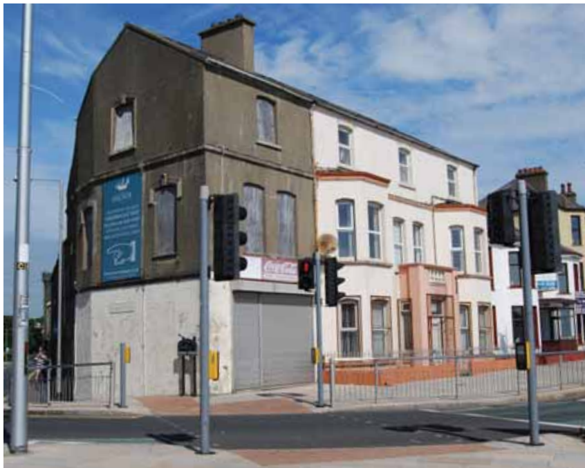
Current derelict properties
