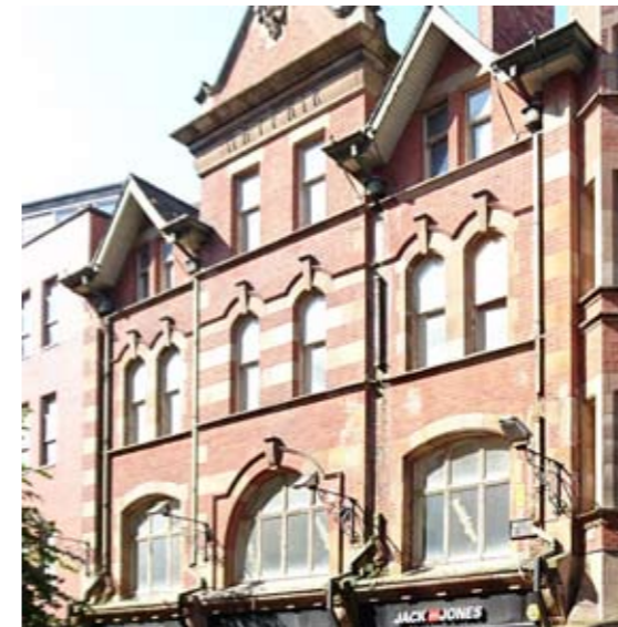
Can you spot the functional downpipes in this photograph of a Grade B1 listed building in the Belfast City Centre Conservation Area? (Clue - there aren't any)
