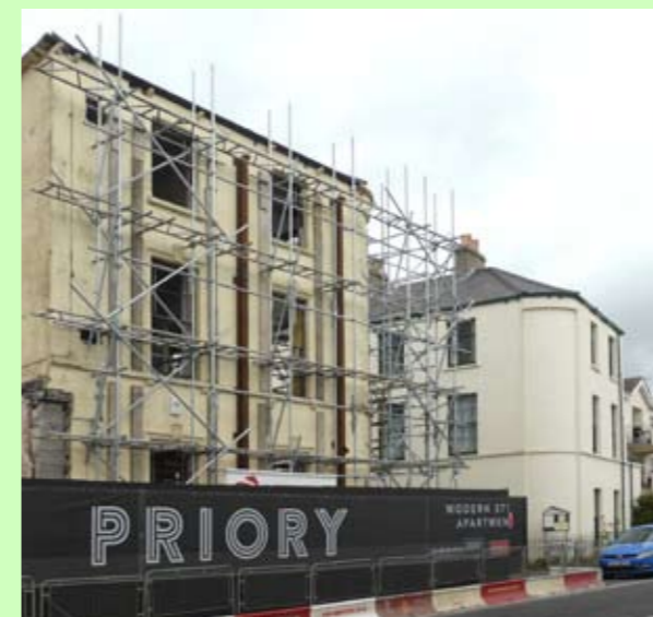
No.1 Stewarts Place immediately before the collapse (far left), after the collapse (near left) and supported by scaffolding pending its restoration (below), with the previously at-risk no.3 to its right.
