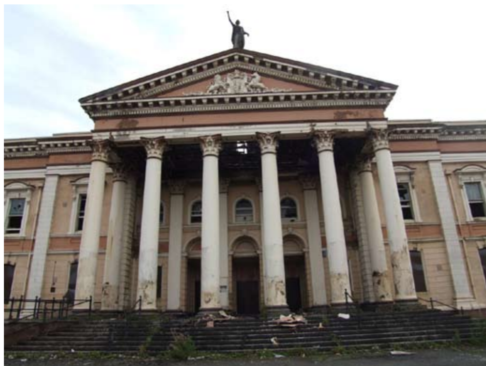
Crumlin Road Court House falling into further decay while currently held in development limbo.
