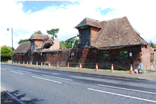
Sion Mills Stable Block (HB10/07/001C - Grade B+) – 2008, before Urgent Works Notice was served
