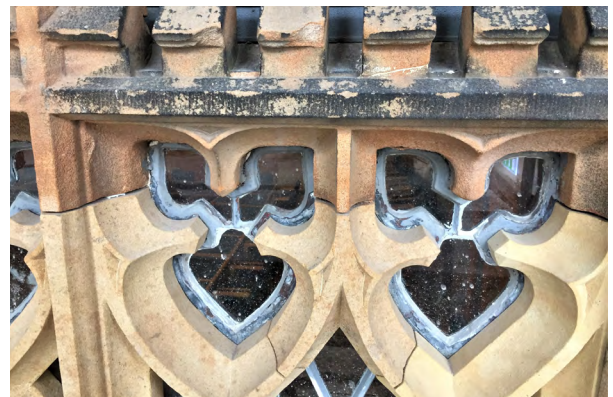
Stone conservation work at The Lanyon Building, Queen's University, Belfast (HB26/27/005 - Grade A)
