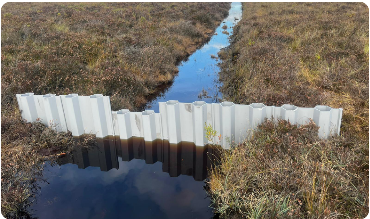
Drain blocking © Ulster Wildlife Trust.
