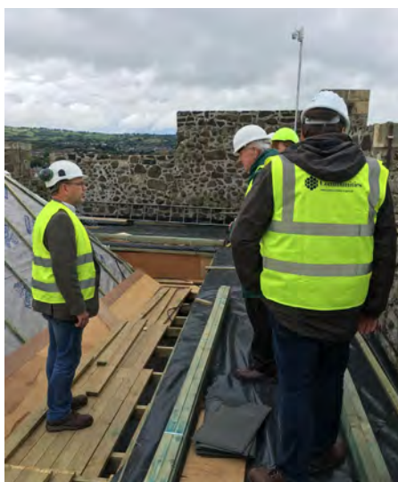
HMC members with Dr John O'Keeffe (HED), visiting the installation works for the new roof at Carrickfergus Castle, a monument in the care of the Department for Communities
