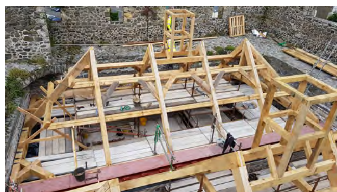
The new roof on the Great Hall at Carrickfergus castle, supported by an Irish oak framework
